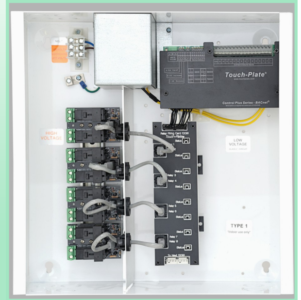
BACnet 8 Relay Panel with Internal I/O Pictured Above in New Enclosure
